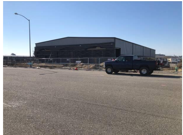
Photo #16 View of the adjoining southern warehouse (31 Richard Brann Drive) currently under construction.
