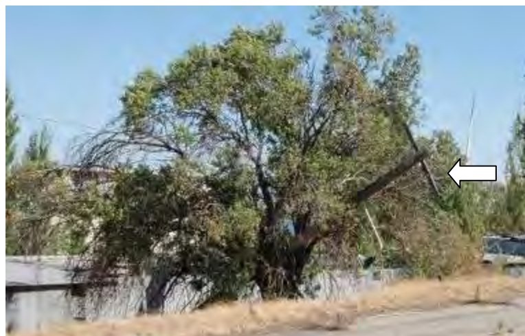
Damaged Electrical Infrastructure
