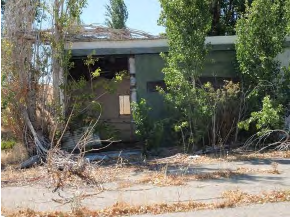
Facility 5: Hazardous Material Storage
