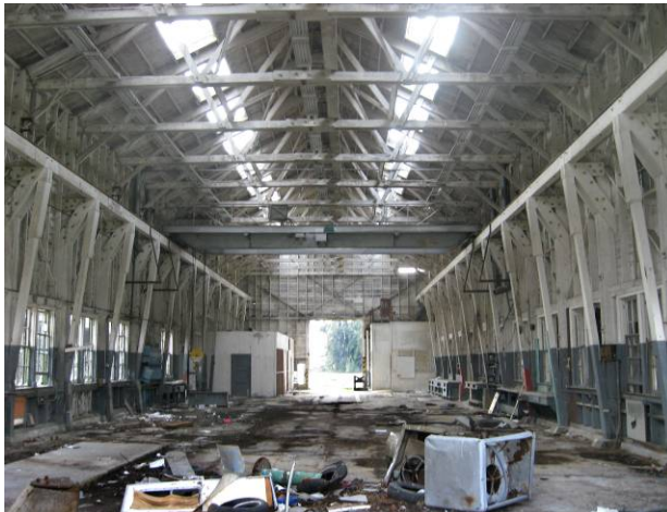
Photo 7. T-11 Ship repair shop interior, unsecured and unsafe, with debris, and distinctive roof trusses.
