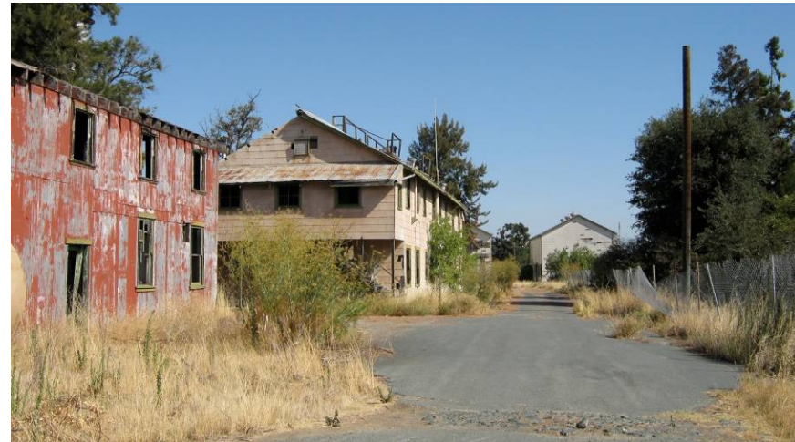
Photo 4. Looking north. Buildings T-27 and T-26 are to the left. Building T-9 is ahead. Dilapidated, unsafe conditions are evident.
