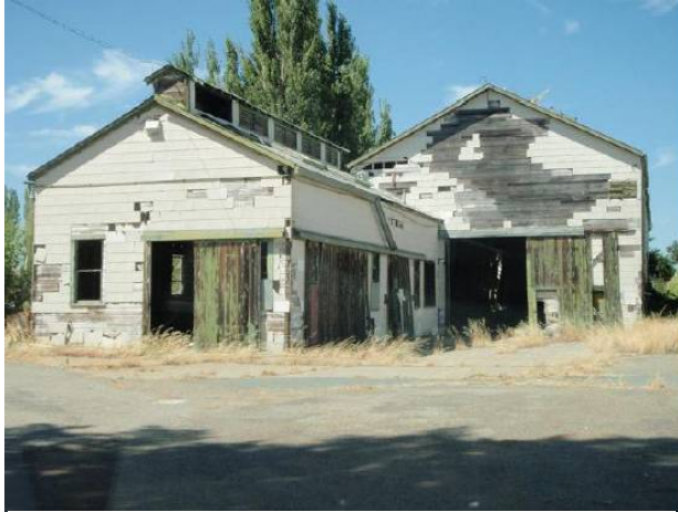
Photo 5. Looking north. T-11 Ship repair shop in dilapidated conditions with damaged exterior materials and faulty weather protection.
